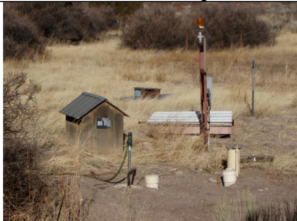
13. House well head and underground pressure tank
