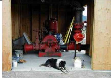
12. Fairbanks Morris pump and PSI relief valve
